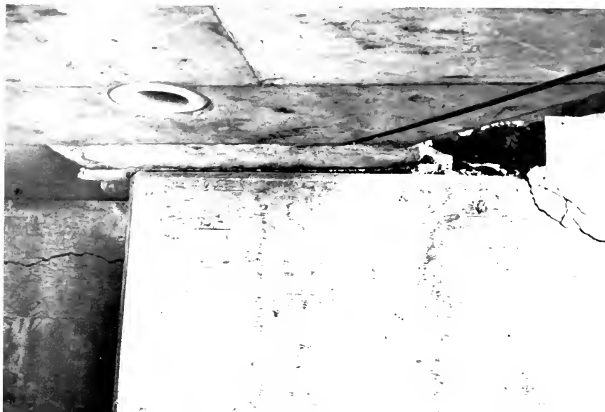
Photo 8. View showing horizontal displacement of bridge deck on its support, San Fernando Road overhead [2].
